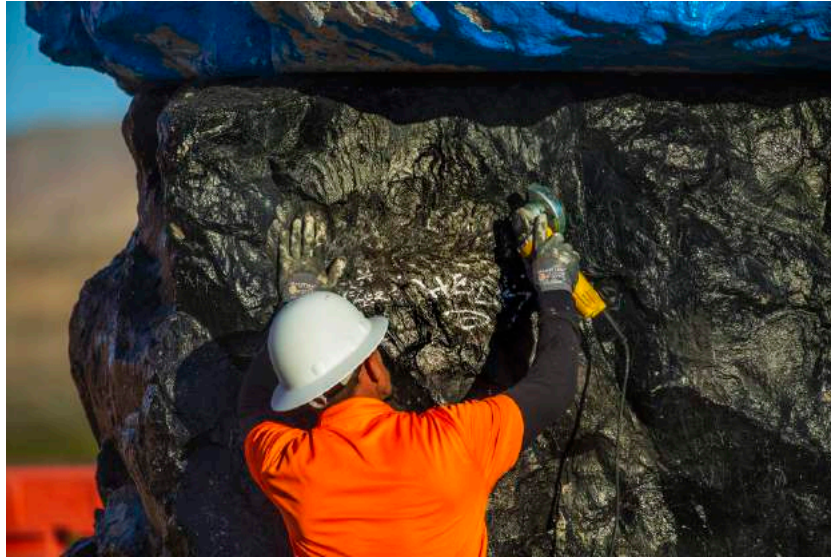
Some graffiti has to be removed with power tools, as John Henderson of Vergith Contracting Co. is seen doing here. After cleaning, a coat of white primer is applied.
