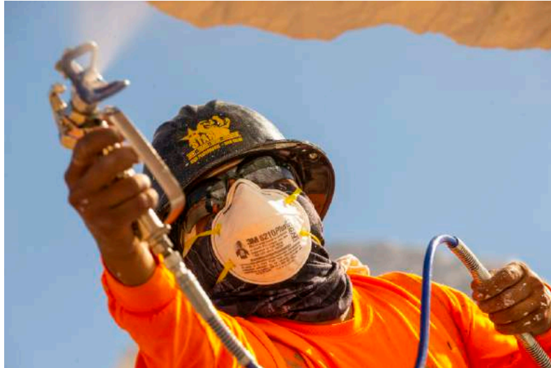
Jose Cervantes with Vergith Contracting Co. evenly sprays a white finish on one of the rocks during the three-week renovation, which took approximately 300 hours to complete
