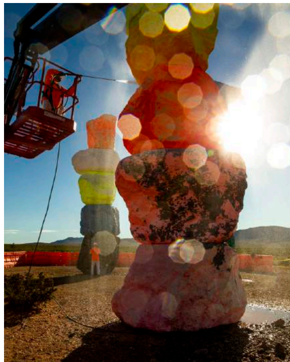
Ivan Ibarra pressure washes a tower after a week of high winds and other safety concerns delayed renovation efforts.
